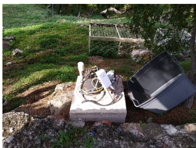
Figure 5: Vault for the 5TDE with plinth made of concrete for improved coupling and Wi-Fi extender.
