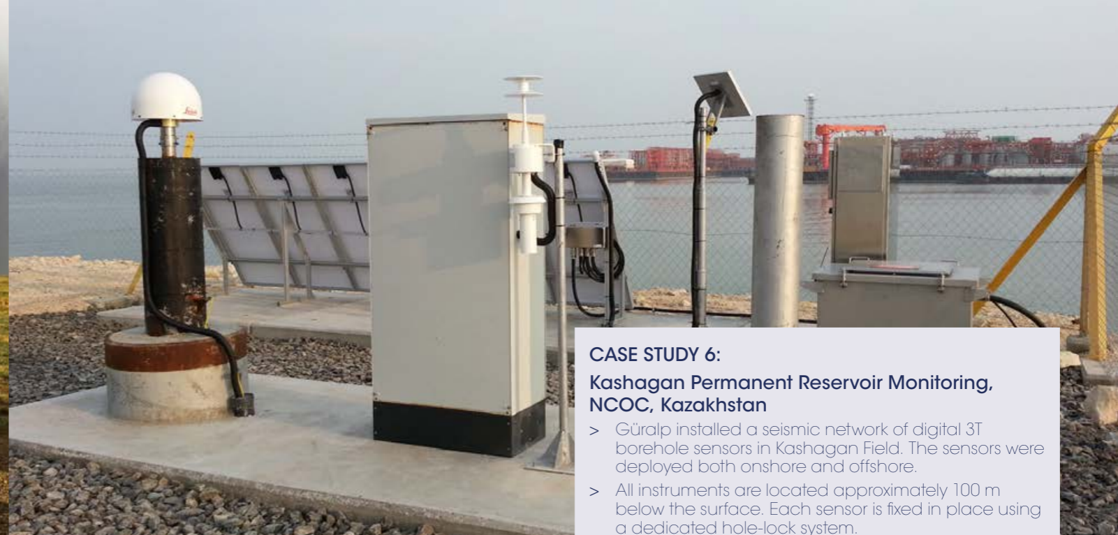
IMAGE 3: STATION INSTALLATION IN KASHAGAN
